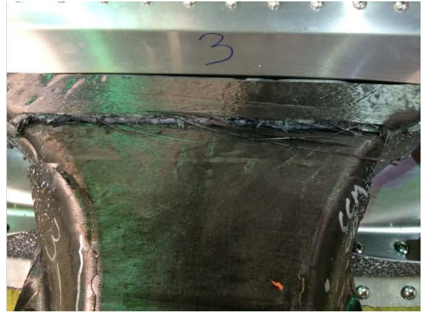
(b) Damage at the Hat Root
