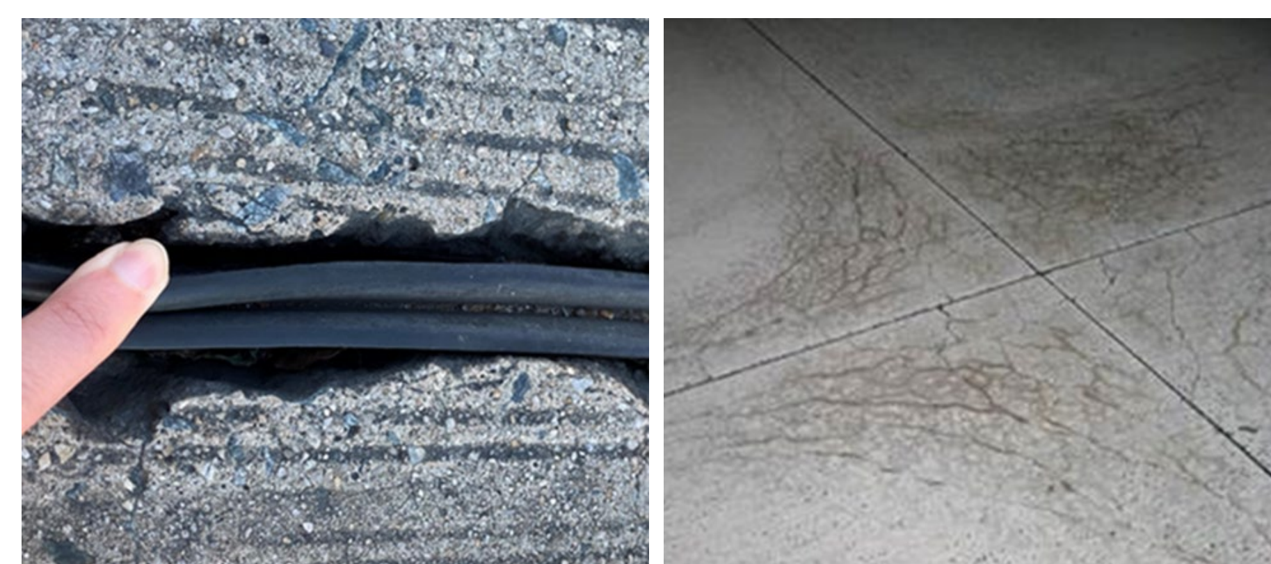
Debonding from concrete
