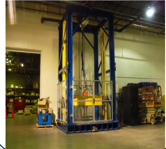
Tower of Power (8/7/09)
