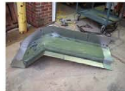
Once the bagging flanges have been tack welded into place, its ready for filling.
